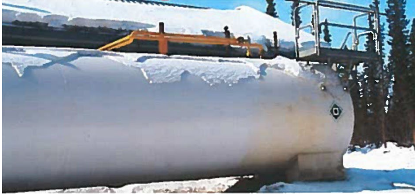
Figure 3 – One 35,000 L diesel fuel tank.
