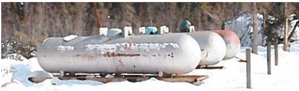
Figure 4 – Three 4,500 L propane fuel tanks.
