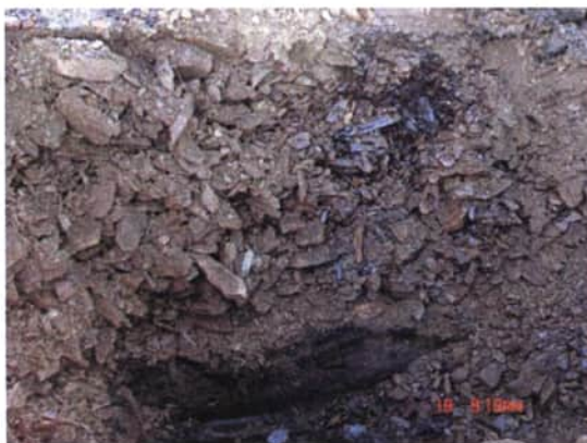
Photo 9 : Tar found in fill material at 02-TP06-04.
