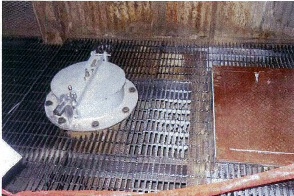
Photo 15 – Pump and Sample hatches
