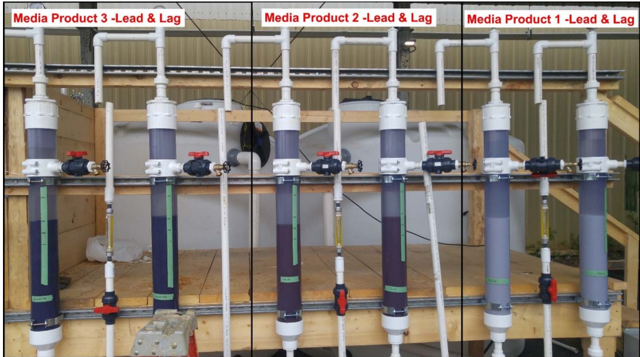
Figure 2-6: Photograph of the Arsenic Removal Contactors
