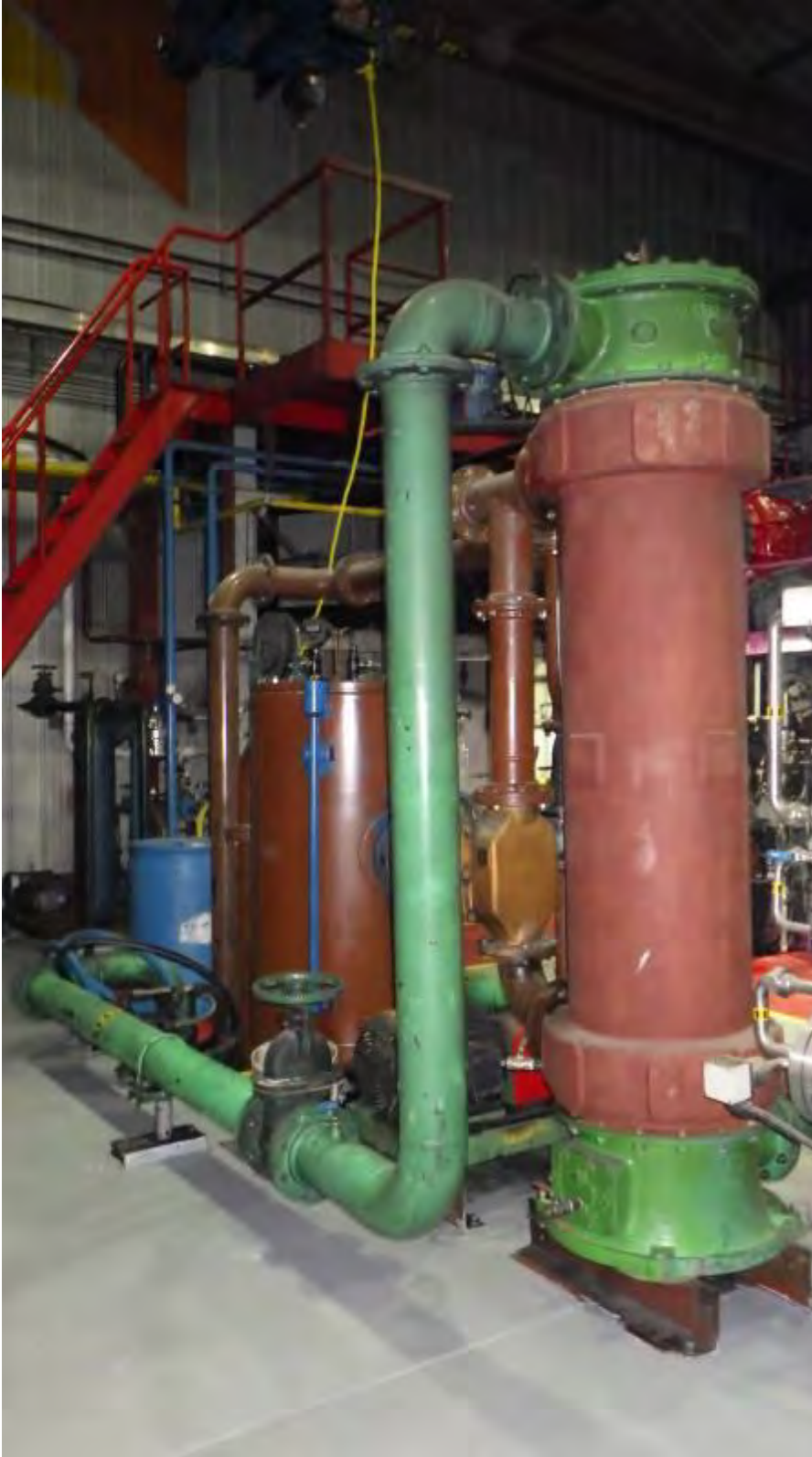
Photo 3: K-Plant Sheet and Tube Oil Heat Exchanger
