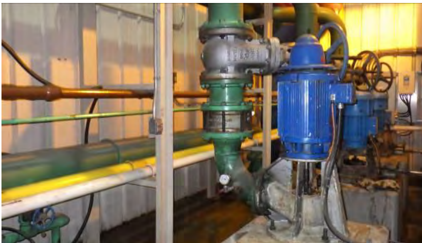
Photo 5: CAT Plant Raw Water Pumps
