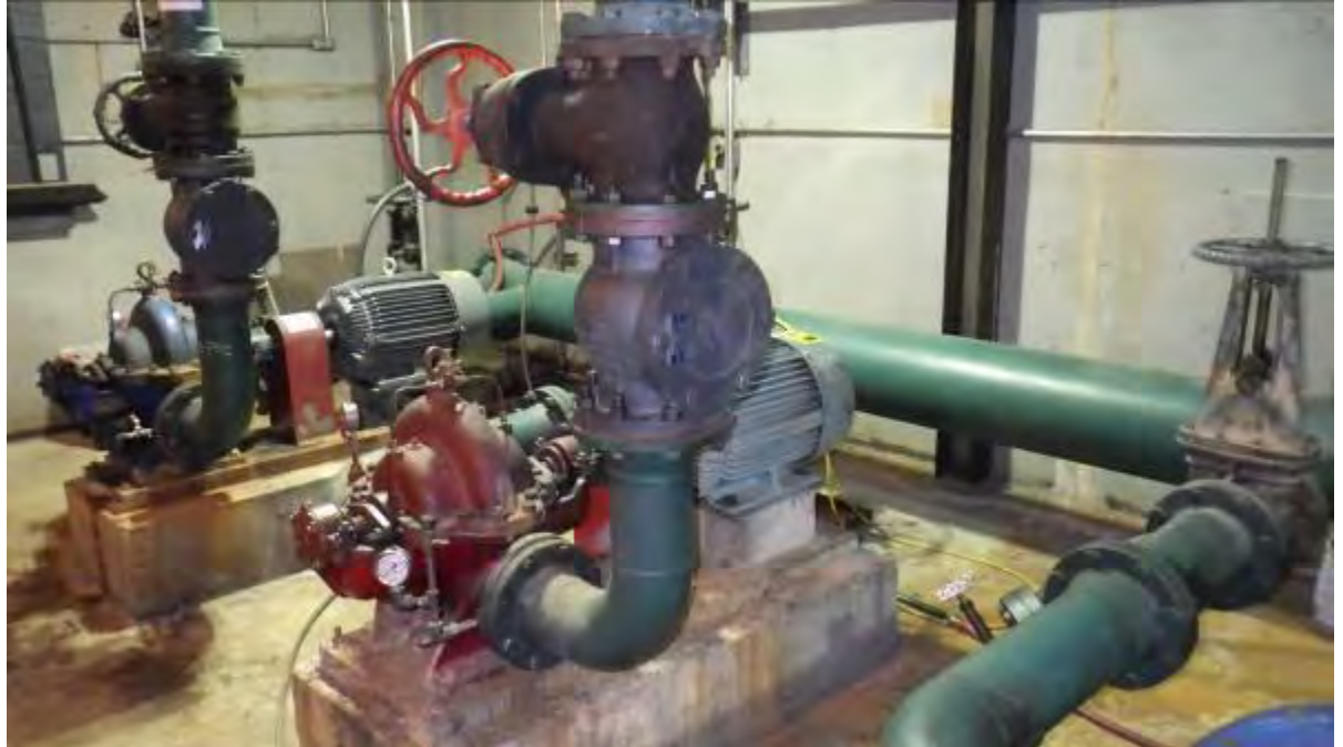
Photo 4: EMD Plant Raw Water Pumps
