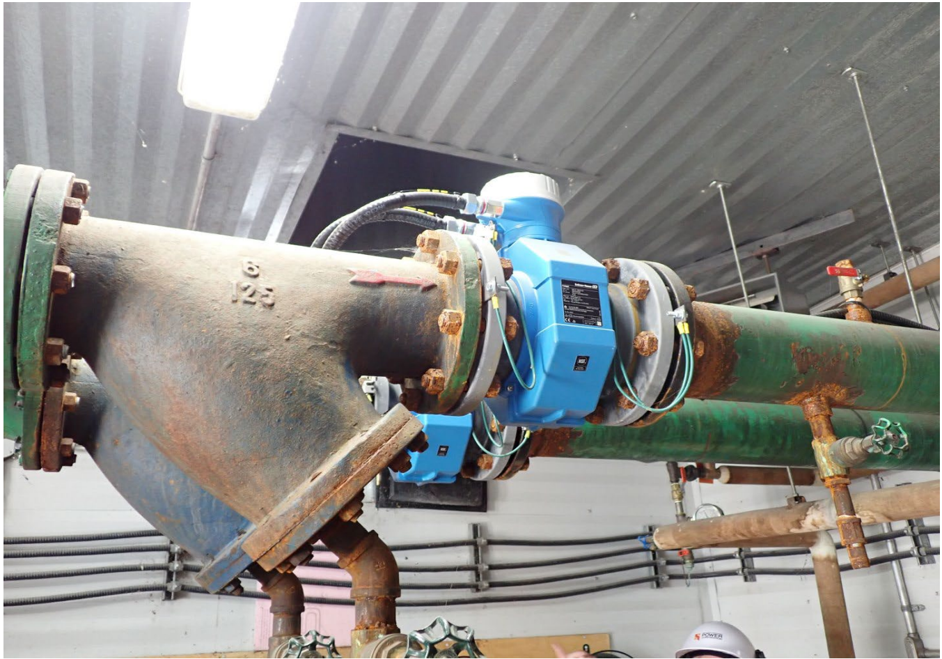
Figure 1 - Example of flow meter to measure water use
