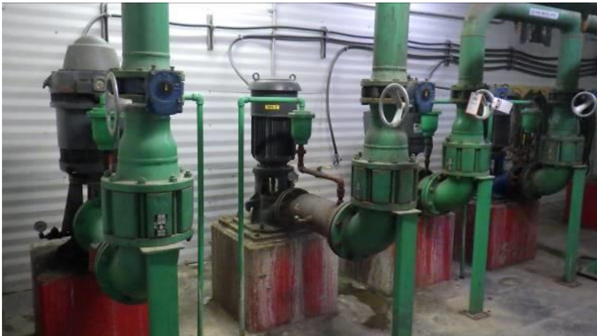
Photo 2: K-Plant Raw Water Pumphouse
