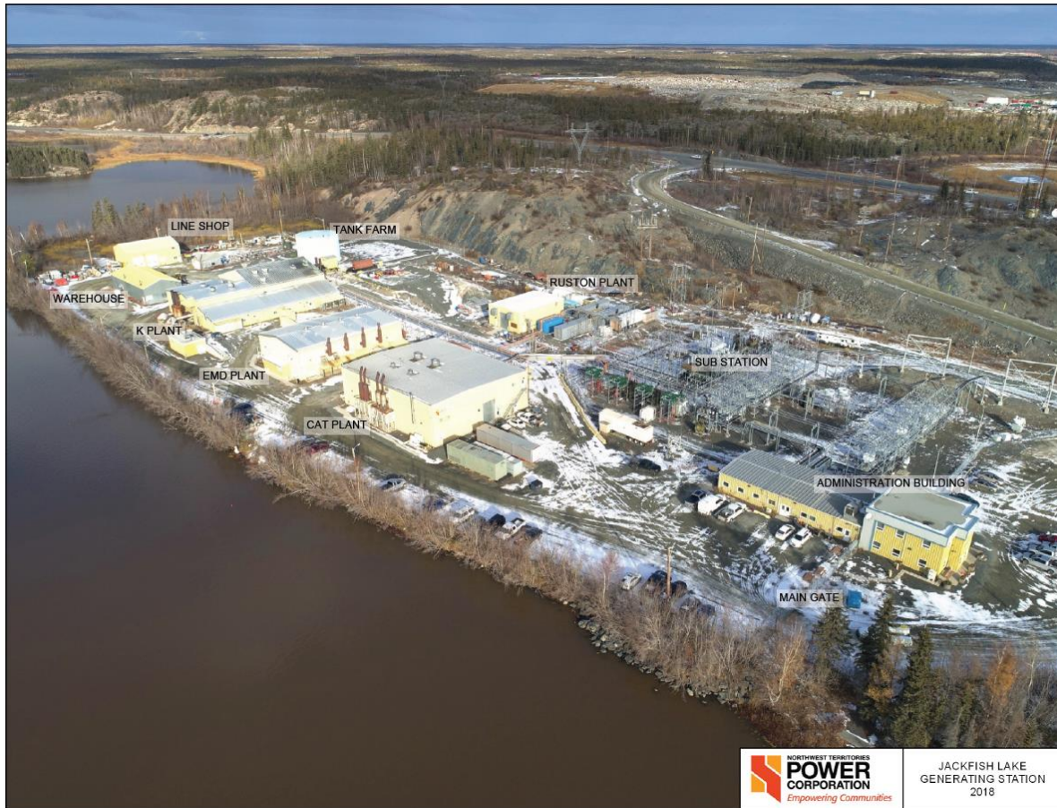
Figure 3: Jackfish Diesel Generating Facility
