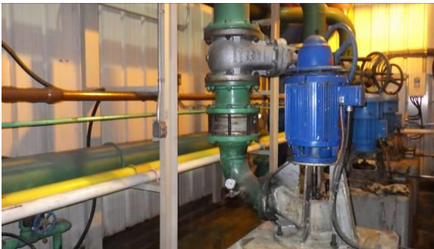
Photo 5: CAT Plant Raw Water Pumps
