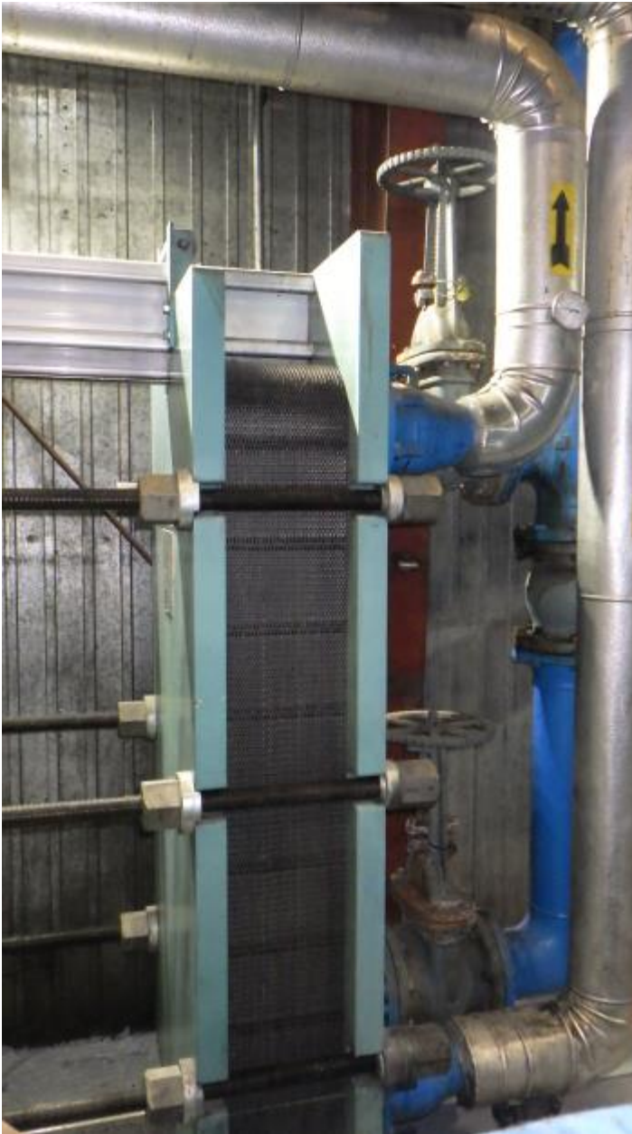
Photo 6: K-Plant Plate Heat Exchanger
