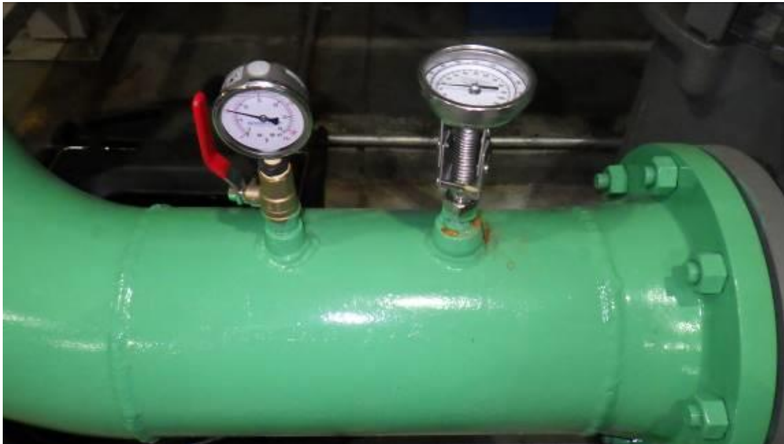
Photo 8: Raw Water Pressure and Temperature Gauges
