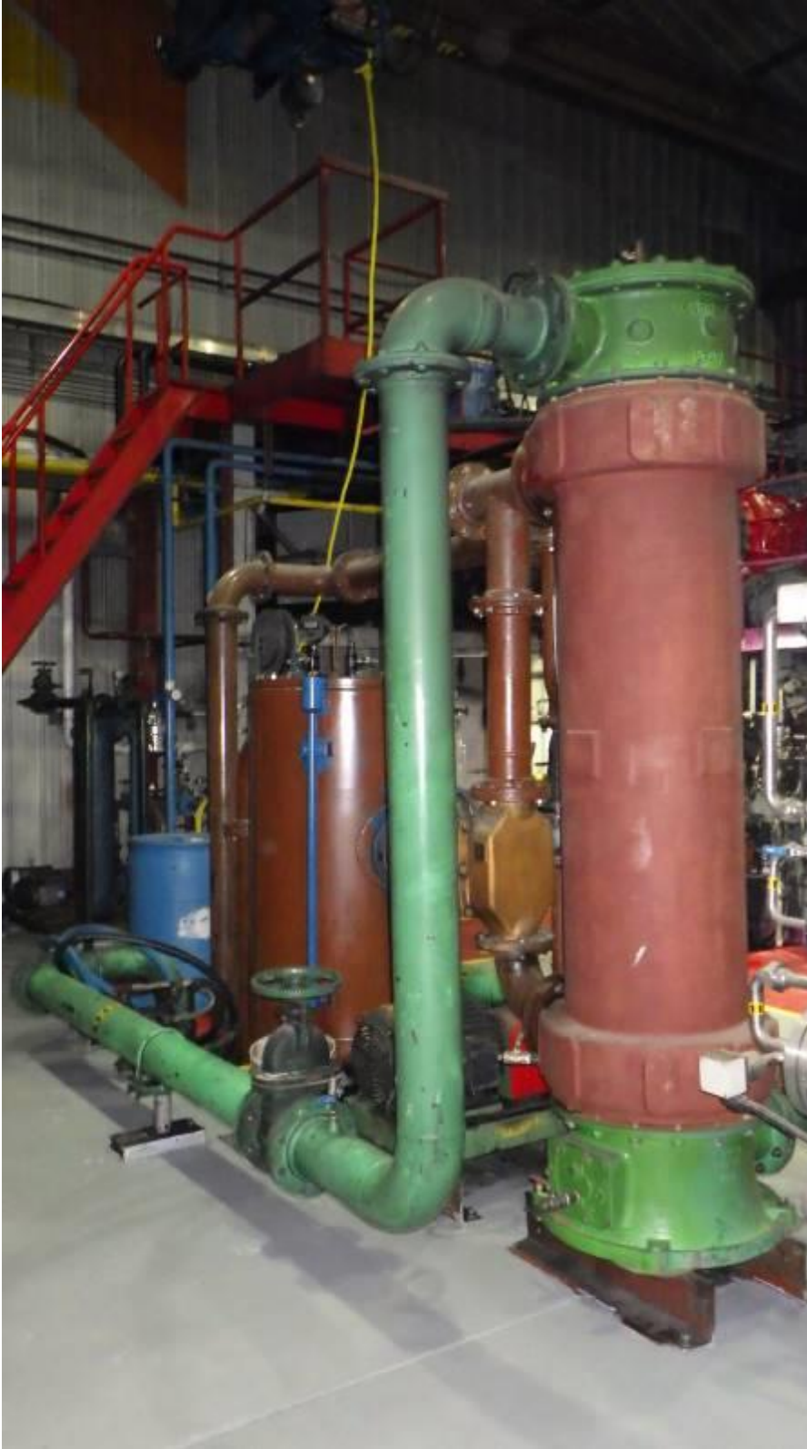
Photo 3: K-Plant Sheet and Tube Oil Heat Exchanger
