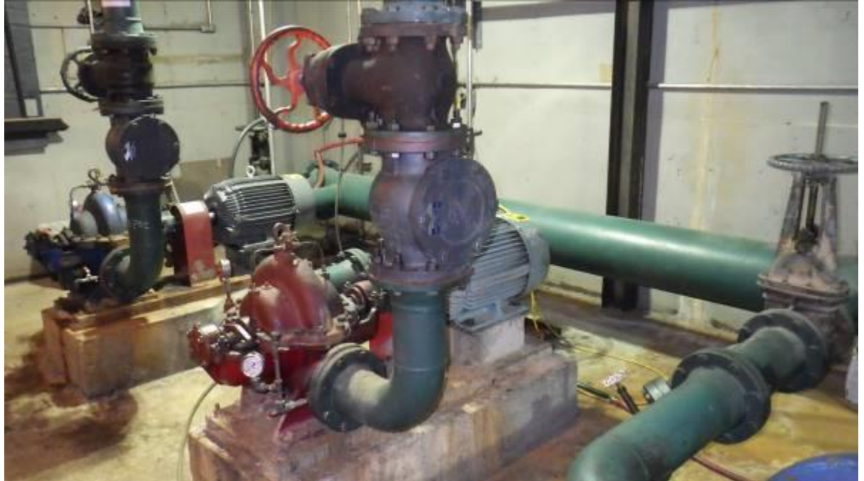
Photo 4: EMD Plant Raw Water Pumps
