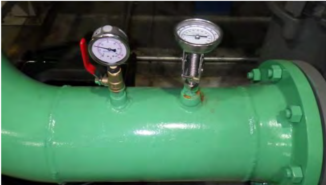
Photo 8: Raw Water Pressure and Temperature Gauges
