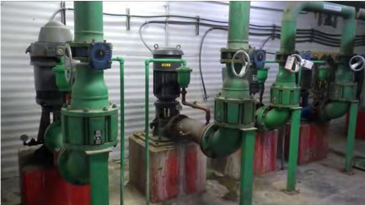
Photo 2: K-Plant Raw Water Pumphouse
