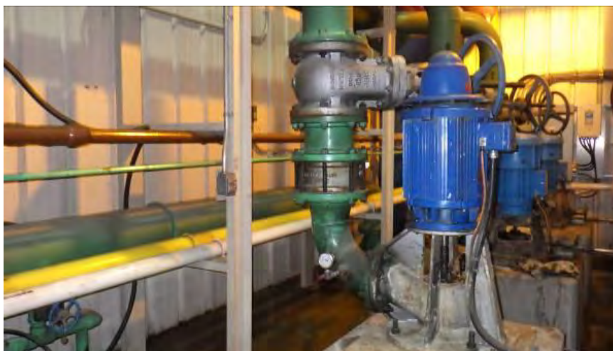
Photo 5: CAT Plant Raw Water Pumps
