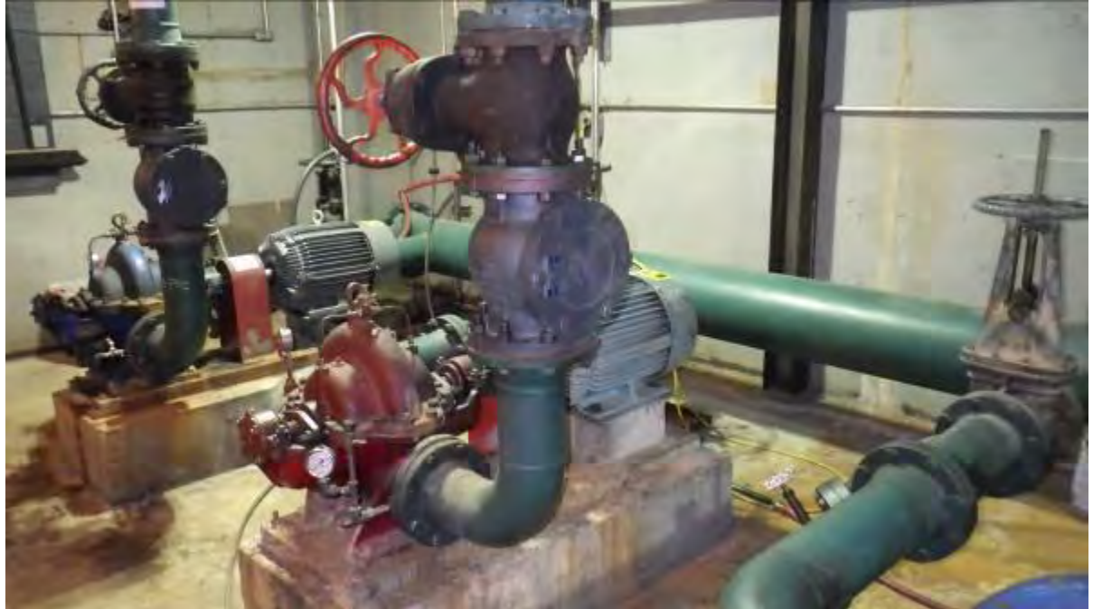
Photo 4: EMD Plant Raw Water Pumps
