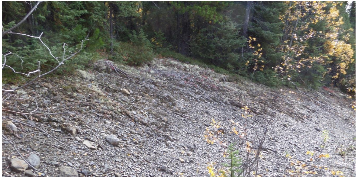
Figure 44: The existing cut slope at BP70. The weathered face appears to be colluvium shale because of the residual fragments left in place, but the slope is in sandy materials.
