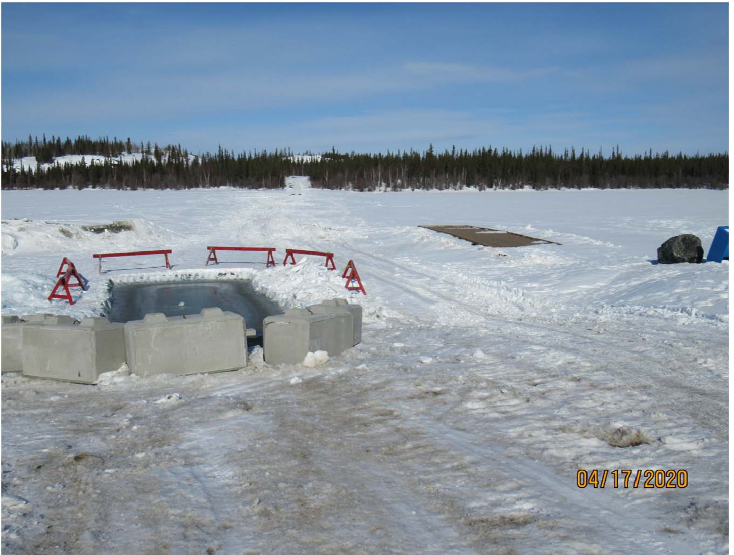
Photo #1 - MV2019X0008 - GNWT-ITI - Prosperous Lake Territorial Park Looking west at the newly installed boat ramp and existing infrastructure at the Prosperous Boat Launch.
