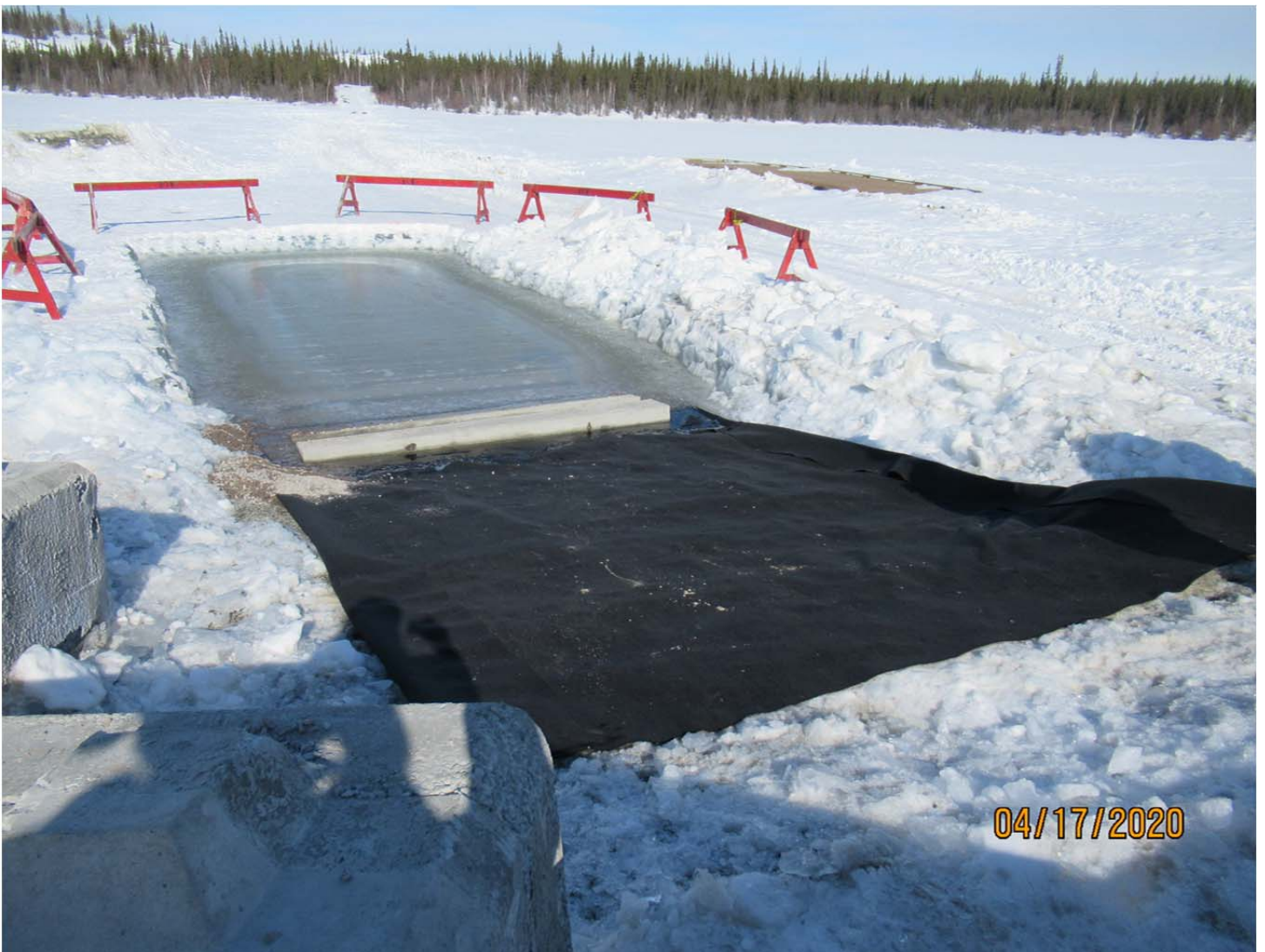
Photo #2 - MV2019X0008 - GNWT-ITI - Prosperous Lake Territorial Park Geotextile fabric and concrete boat ramps have been installed south of the existing ramp & dock.
