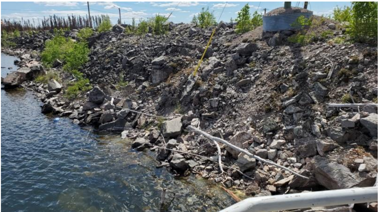
Photo 13. Shows the upstream face of the dam left of the intake. The slope is steep and without adequate erosion protection. The power pole caisson is also undermined. It is recommended that riprap improvements be carried out and the power pole be adequately supported.
