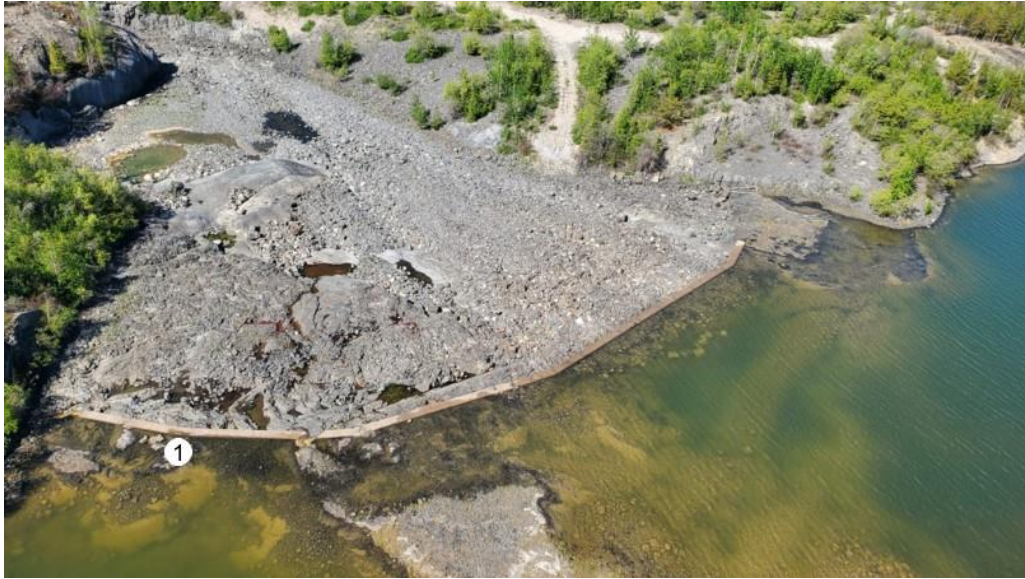
Photo 33. Shows the Forks Overflow Spillway Weir. Repair to weathered concrete at the crest was carried out in 2024 at location (1)
