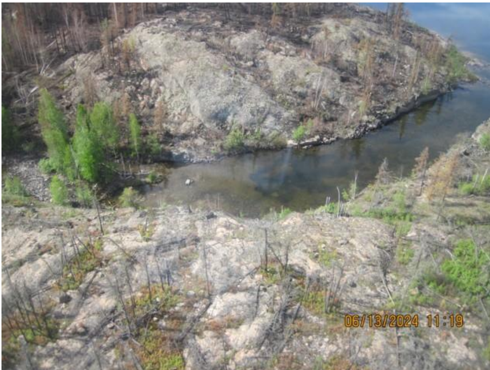
Photo 18. Shows the spillway channel at location 2. There is no concrete sill.
