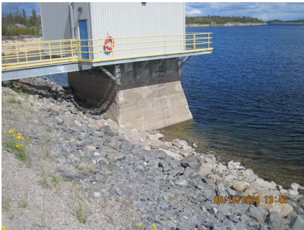
Photo 20. Intake at Rapids Dam. Some surface weathering of the concrete.
