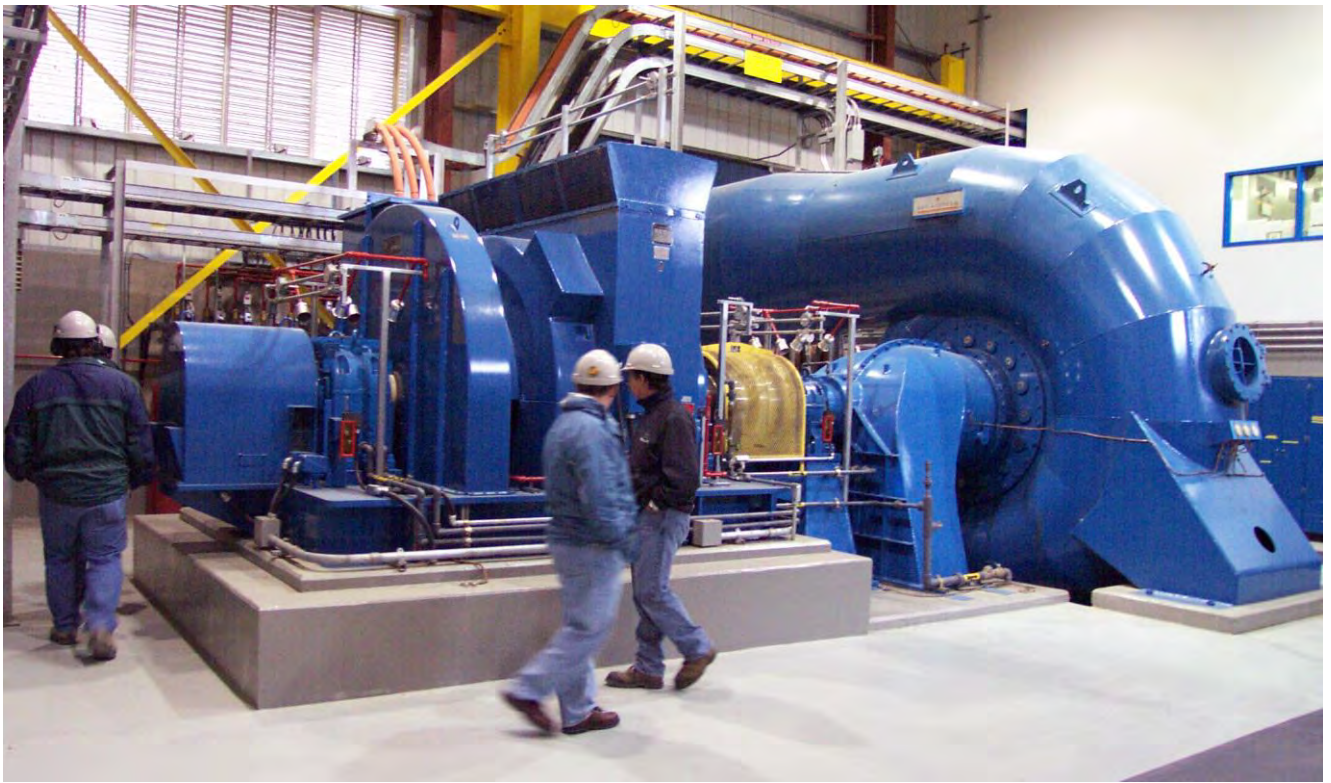
Figure 8: Bluefish Generating Unit # 2 (Plant #2)
