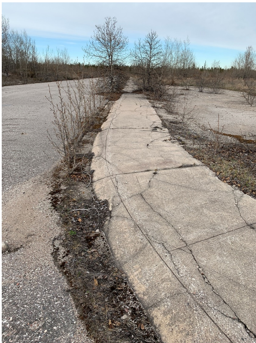
Photo 4: Remaining Street and Sidewalk at the Pine Point Townsite
