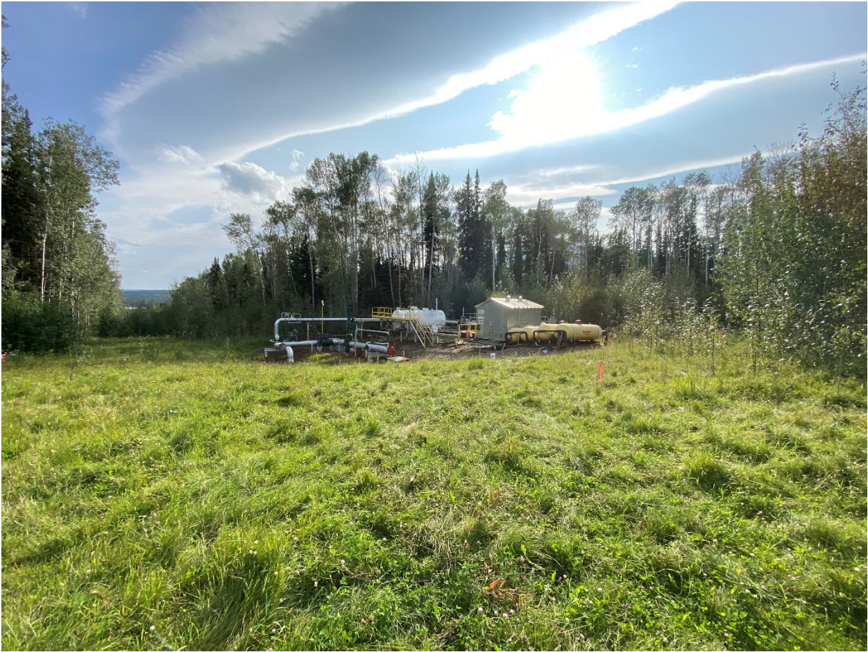
Photograph 2: Facing southwest towards aboveground infrastructure at PM-1.
