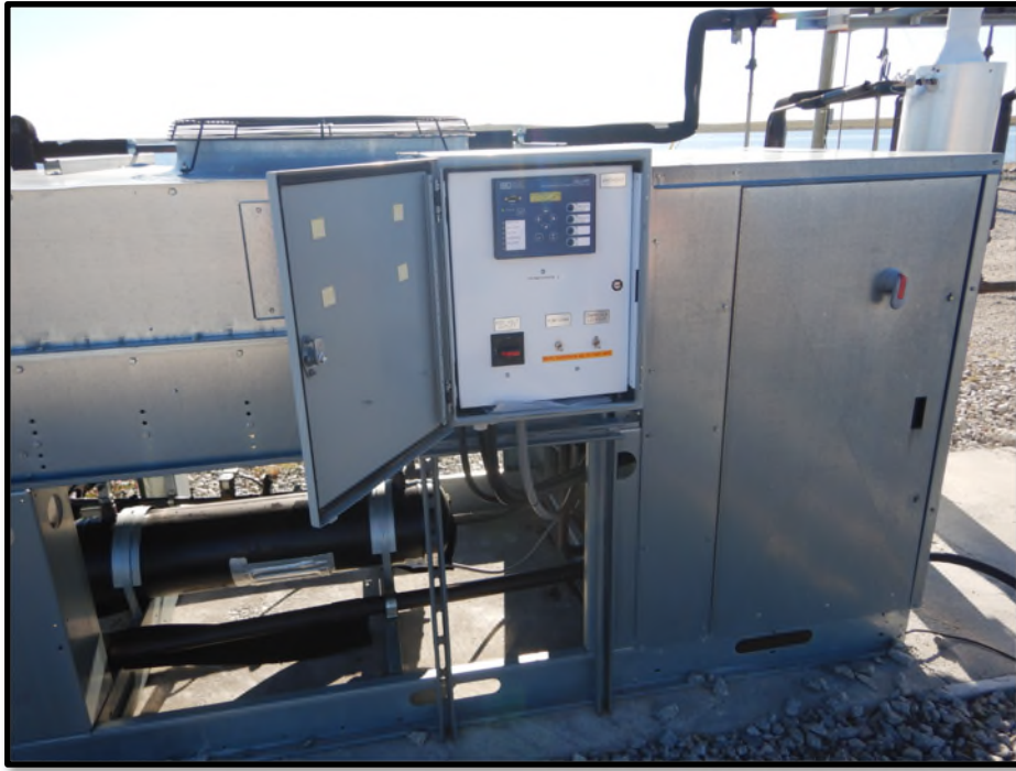
Photo D11: General view of thermosyphon cluster control panel.
