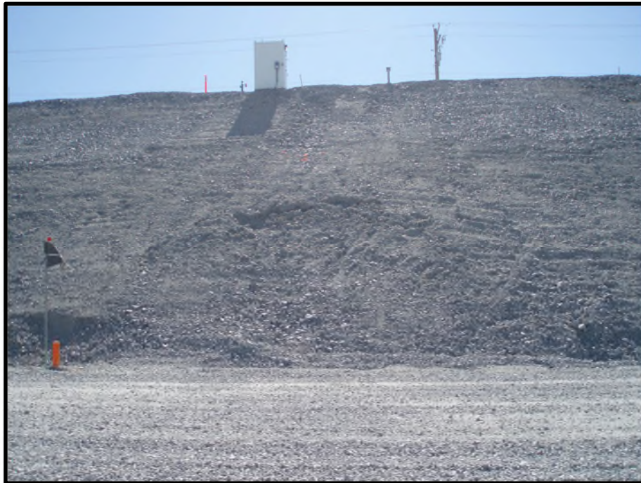
Photo D46: Same downstream slope undulation shown in Photo D45 (photo provided by DDMI from 2007).
