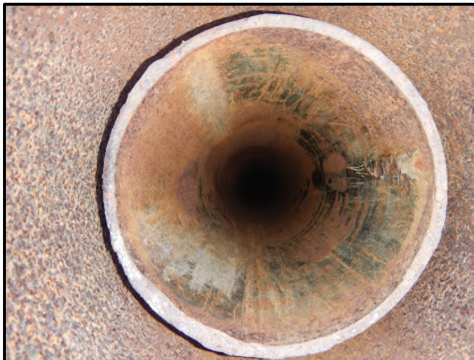
Photo D40: Inactive pressure relief well along the downstream crest.
