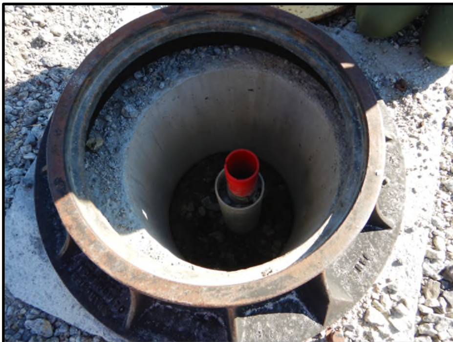
Photo D34: Inclinometer casing within the protective instrumentation housing shown in Photo D33.
