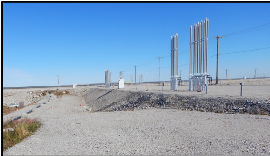
Photo D10: North Island C Thermosyphon Cluster (shown in foreground) and North Abutment Thermosyphon Cluster (shown in background).
