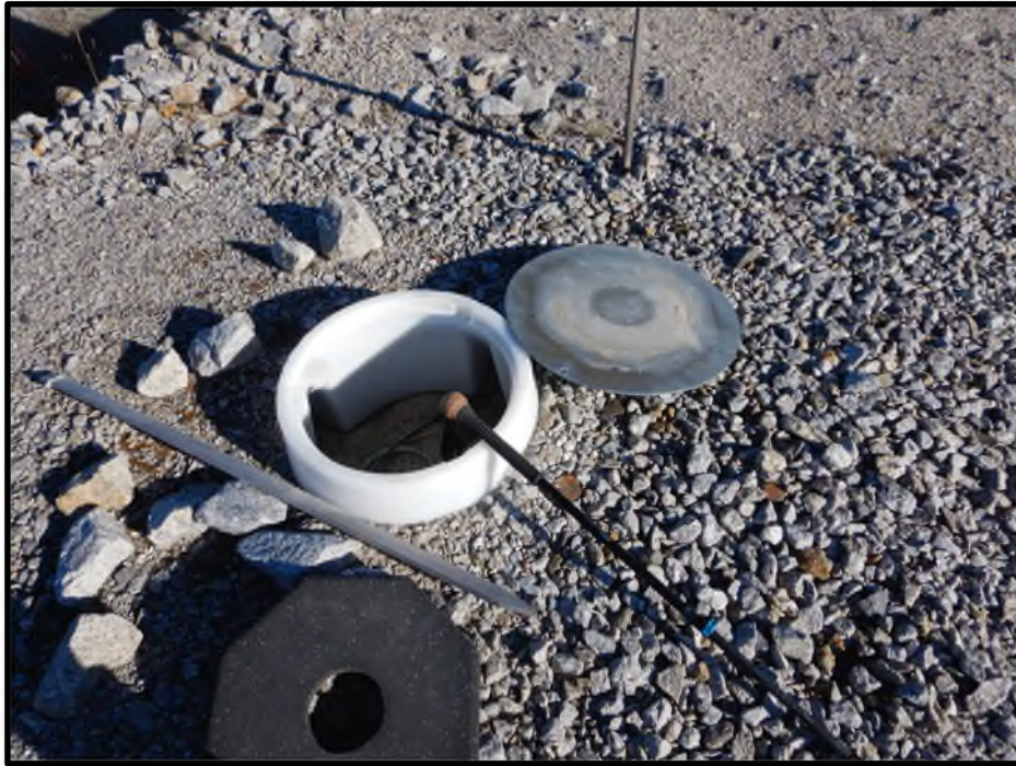
Photo D31: Protective instrumentation housing for vibrating wire piezometers along the downstream crest.
