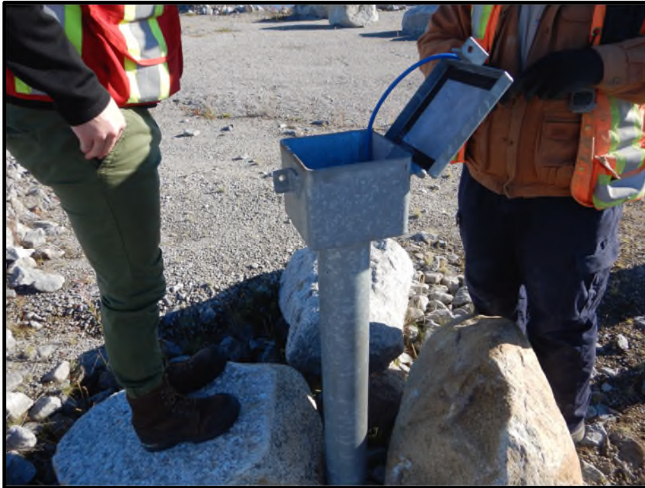
Photo D37: Protective instrumentation housing for a ground temperature cable installed along the top of dike.
