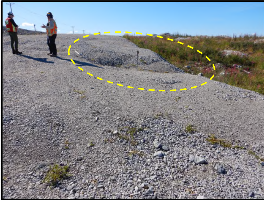
Photo D43: Thaw settlement of upstream thermal berm near Station 0+100.
