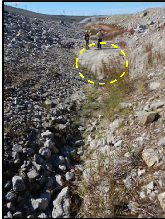
Photo D23: Downstream toe ditch near Station 0+450 showing sediment accumulation upstream of check dam.
