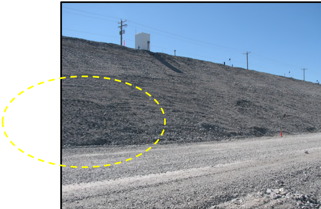
Photo D48: Same downstream slope regrading shown in Photo D47 (photo provided by DDMI from 2007).
