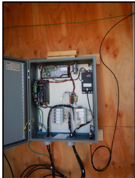
Photo D28: Multi-channel instrumentation data logger within data logger shelter.
