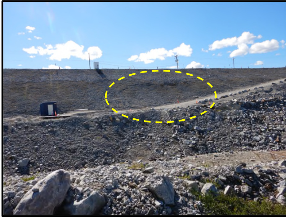
Photo D45: Downstream slope undulation observed near Station 0+900 (photo taken by Tetra Tech in 2022).
