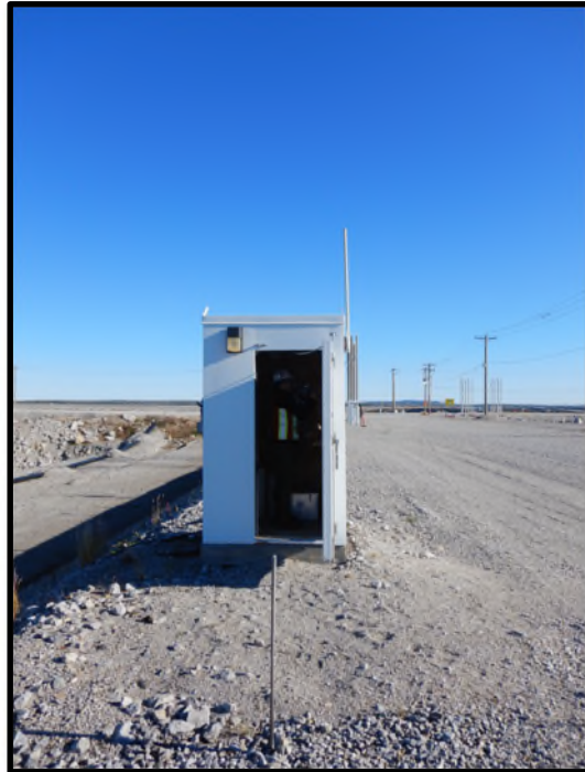
Photo D27: One of three data logger shelters along the downstream crest of the A418 dike.
