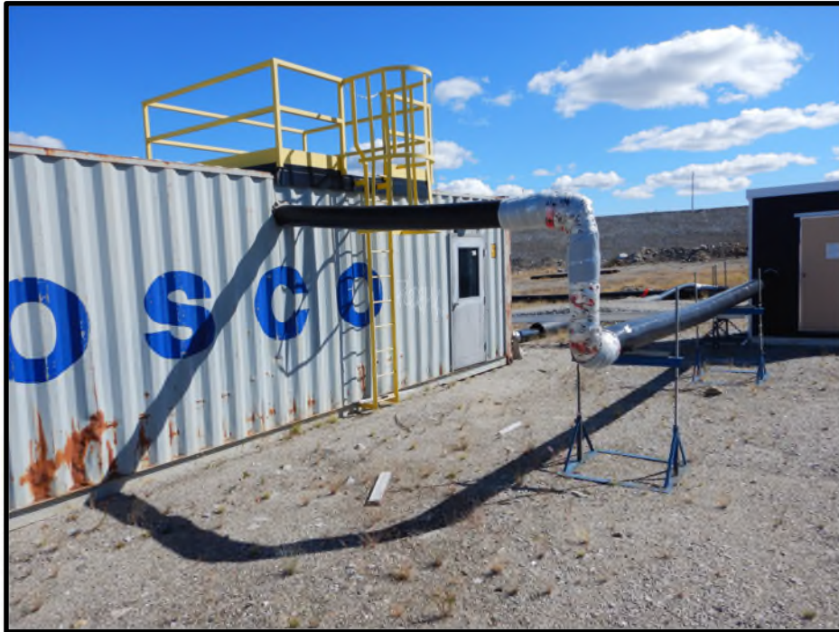
Photo D19: Sea can enclosure for the infield depressurization water collection system and booster pump.
