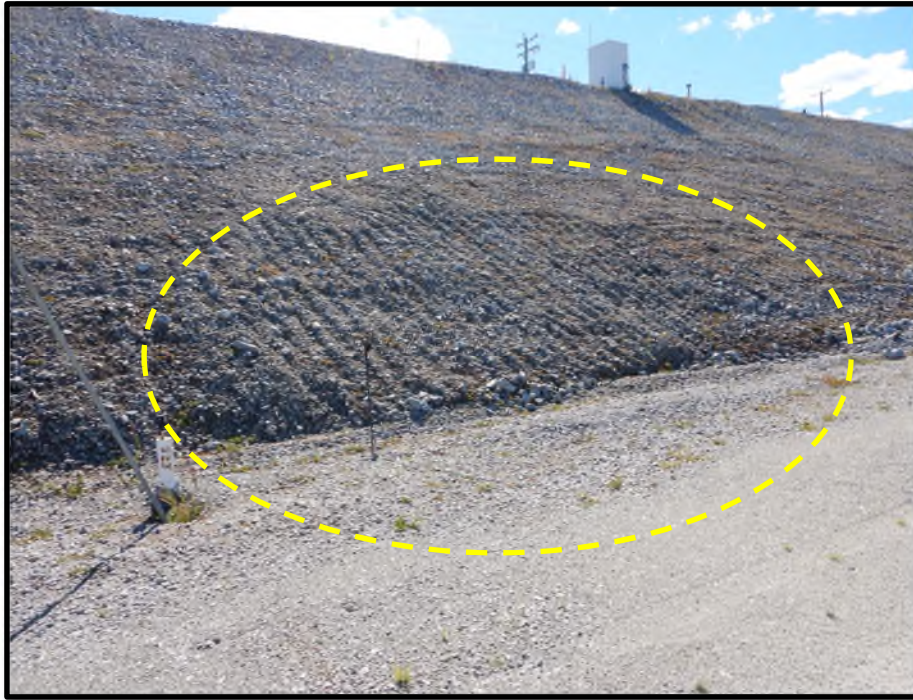
Photo D47: Downstream slope regrading observed near Station 0+575 (photo taken by Tetra Tech in 2022).
