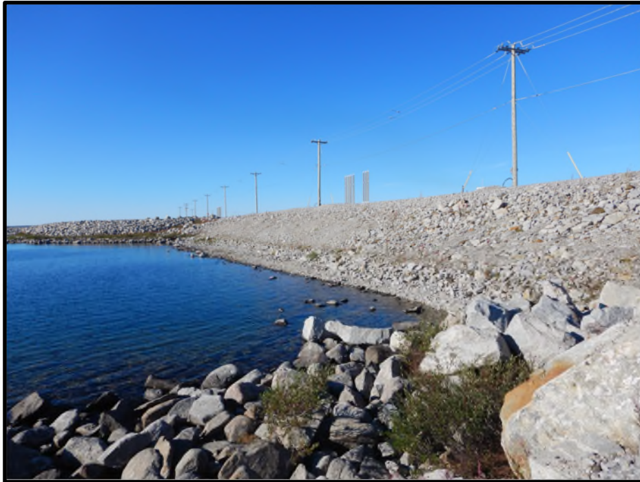
Photo D1: North Abutment upstream slope near Station 0+000, looking south from the A154 Dike.
