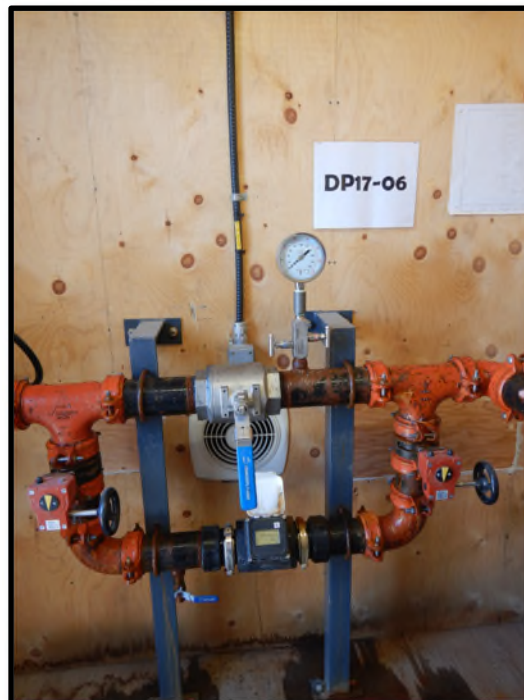
Photo D18: Infield depressurization headers and pipework within protective shelters.
