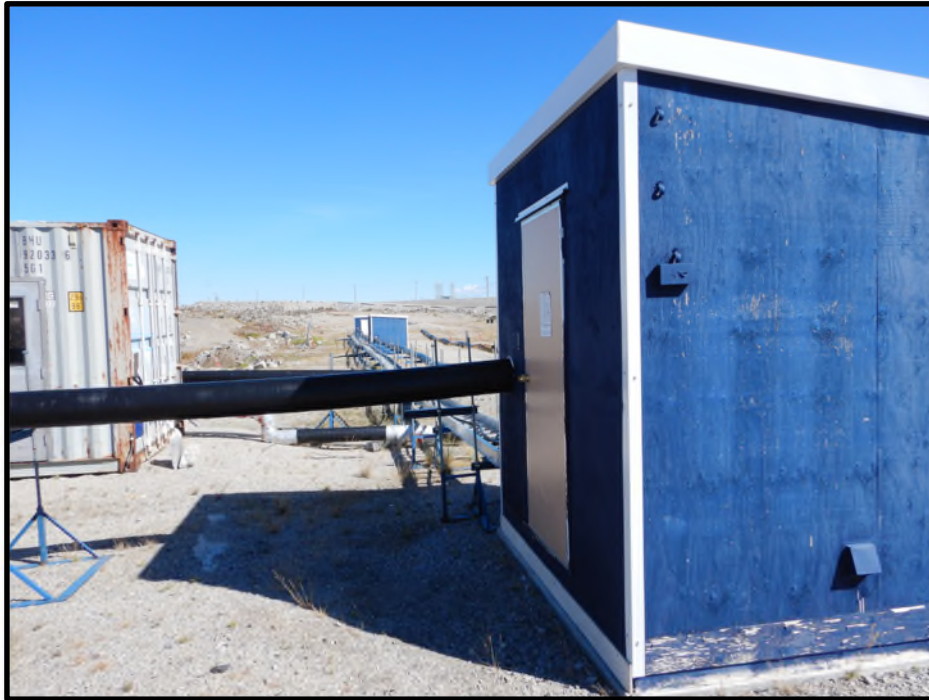
Photo D17: Protective shelters housing the infield depressurization headers and pipework.
