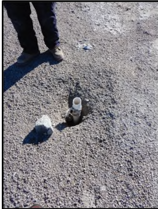
Photo D41: One of nine post-construction in situ density evaluation test holes that were undertaken in 2016 along the upstream crest between Stations 0+550 and 0+850.
