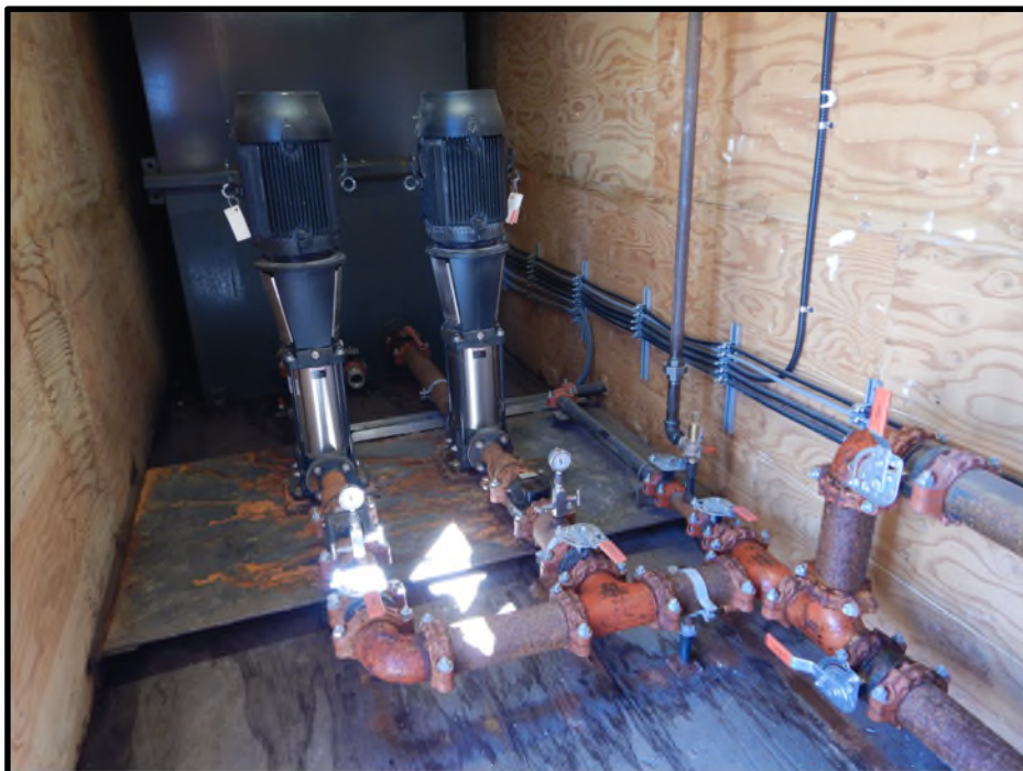
Photo D20: Booster pump and header pipes within the sea can enclosure shown on Photo D19.
