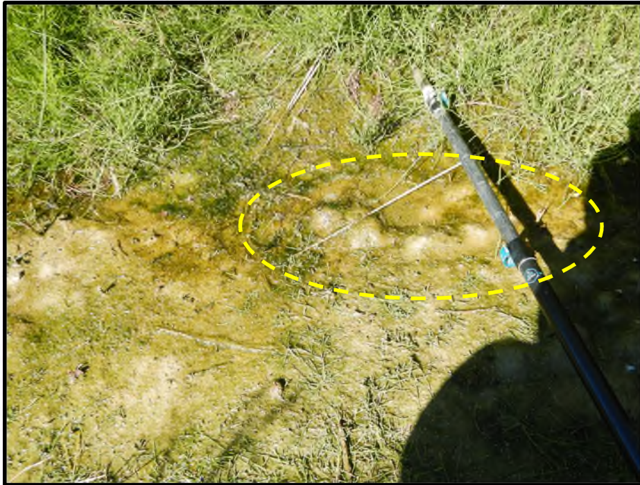
Photo D25: Downstream toe ditch near Station 0+550 showing blisters of air and water found in the ditch sediments.
