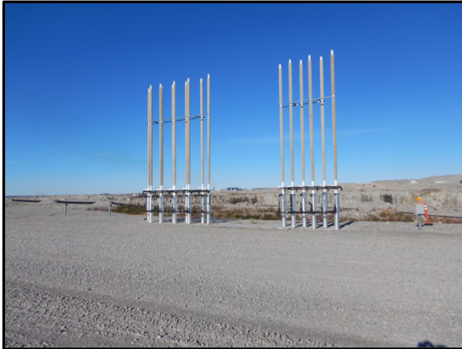
Photo D9: South Abutment Thermosyphon Cluster.
