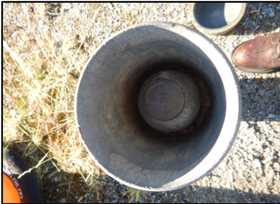
Photo D36: Survey monument within the protective casing shown in Photo D35.
