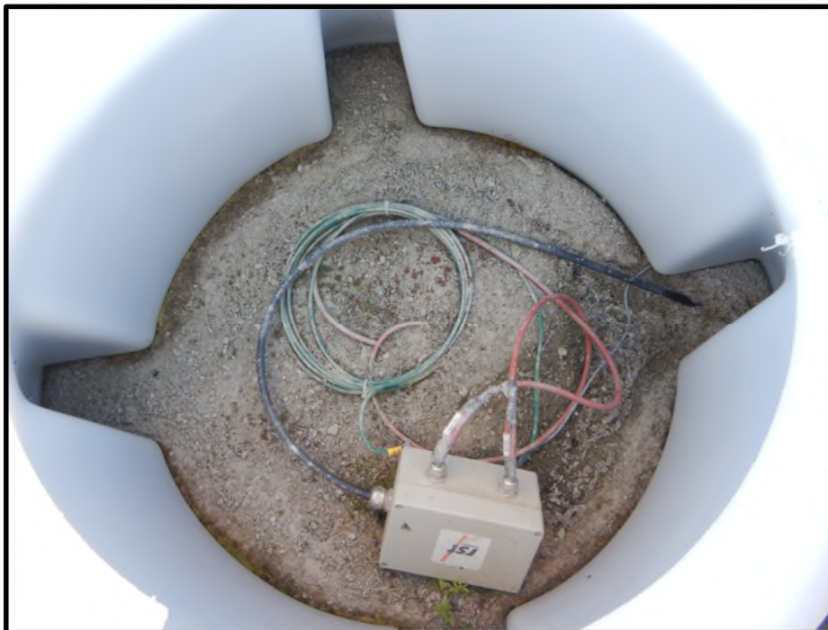
Photo D32: Vibrating wire piezometer junction box within a protective instrumentation housing.
