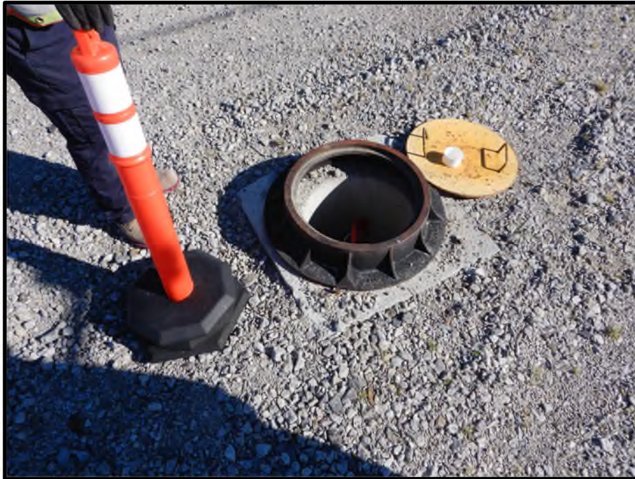
Photo D33: Protective instrumentation housing for an inclinometer along the upstream crest.
