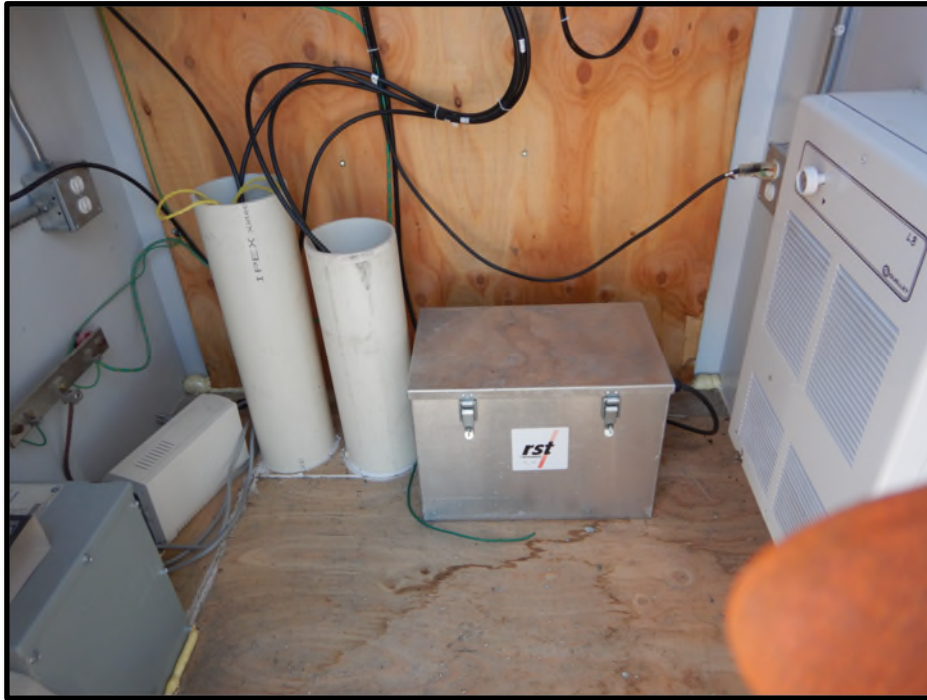
Photo D29: Backup battery pack for multi-channel instrumentation data logger within data logger shelter.
