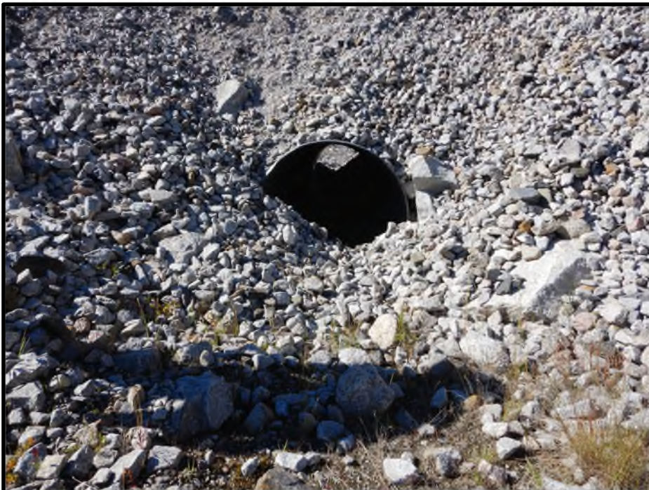
Photo D44: Partially blocked culvert along downstream water collection ditch near Station 0+800.
