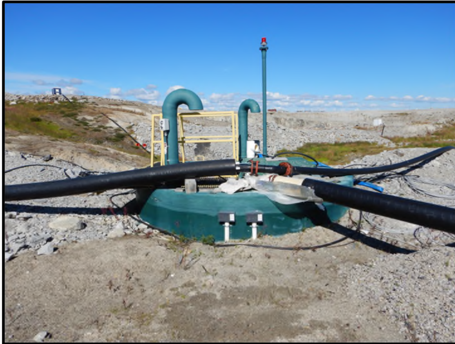
Photo D13: DPS-6 dike pumping station with connected pipelines to relief wells and infield collection sumps.
