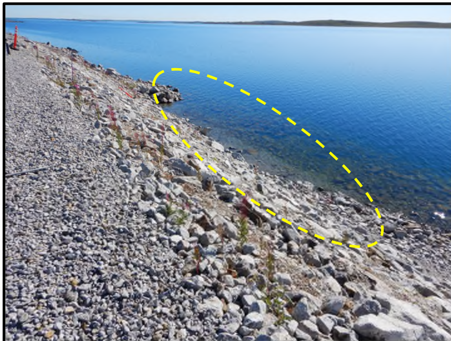
Photo D42: Gap in erosion protection along the upstream slope near Station 0+750.
