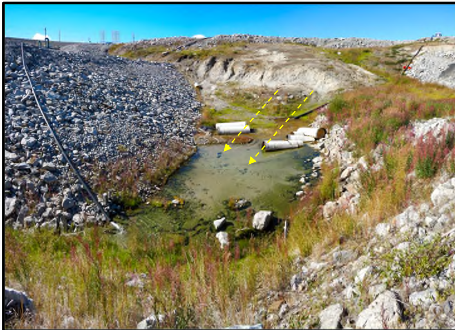
Photo D14: DPS-6 intake pond showing small sinkholes observed at the base of the pond.
