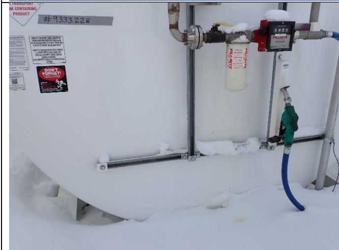
Photo #4: Contaminated snow from dripping liquid at the fuel tanks.
