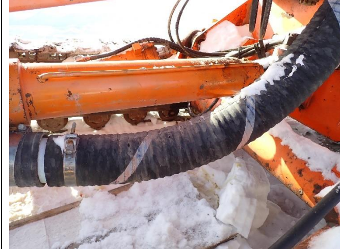
Photo #10: Additional liquid from drilling equipment that has contaminated surrounding snow and must be addressed.
