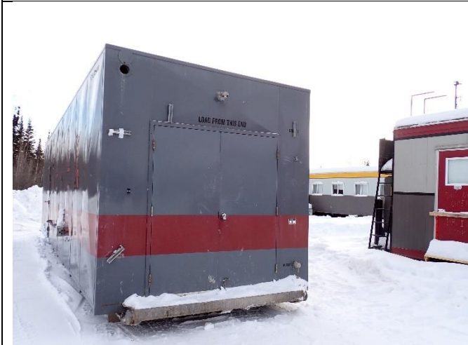
Photo #2: The old wastewater treatment plant that was in operation during the 2024 construction season. This unit will be replaced in 2025 with a larger unit.
