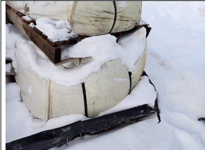
Photo #7: Tear in the side wall of a berm holding waste on site. All secondary containment should be inspected to ensure they function effectively prior to spring melt.
