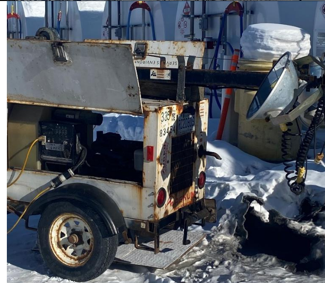
Photo #16: Replaced drip-tray under machinery. Snow staining from light tower exhaust still requires collection and appropriate disposal. Photo provided by Sanexen.
