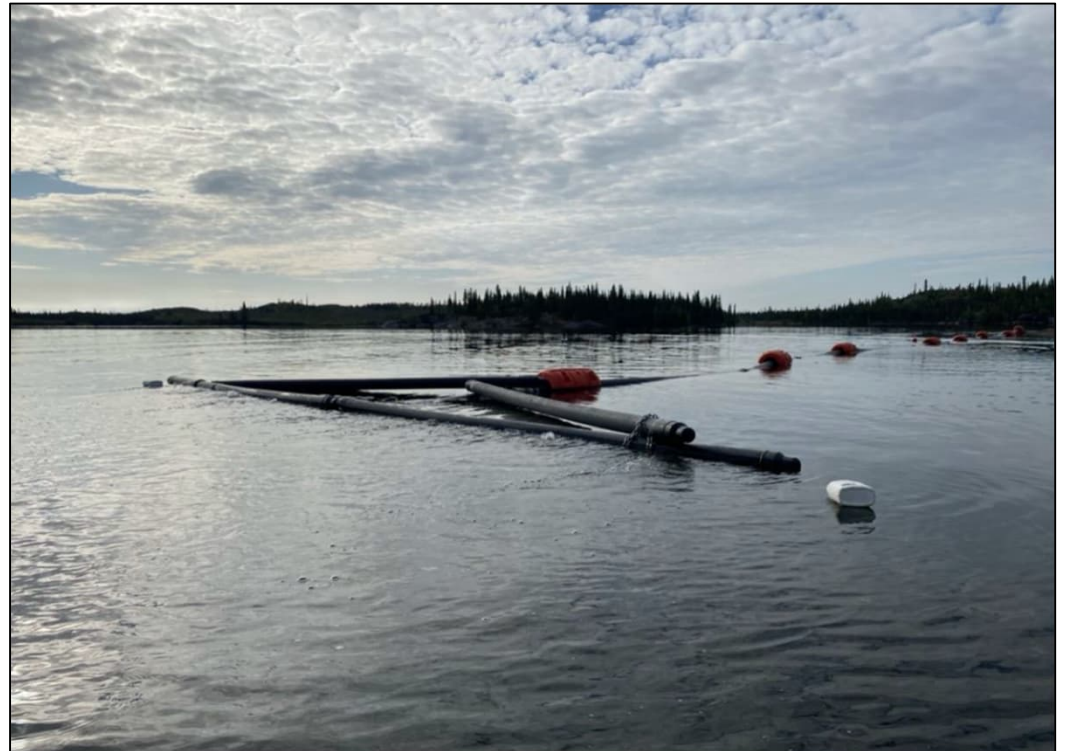
Diffuser operating at end of effluent discharge line to Sherman Lake, August 16, 2024
