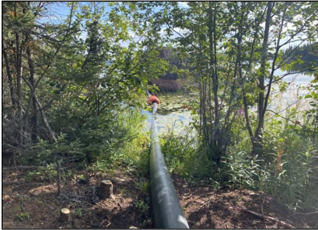
Discharge line to Sherman Lake from shore, August 16, 2024
