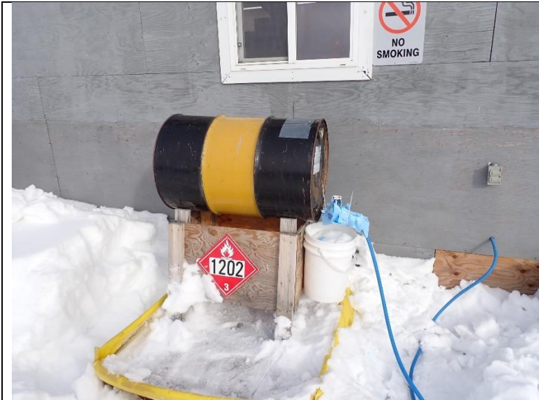
Photo #4: Fuel is stored elevated from the ground, with appropriate secondary containment and cleared of snow on a regular basis.
