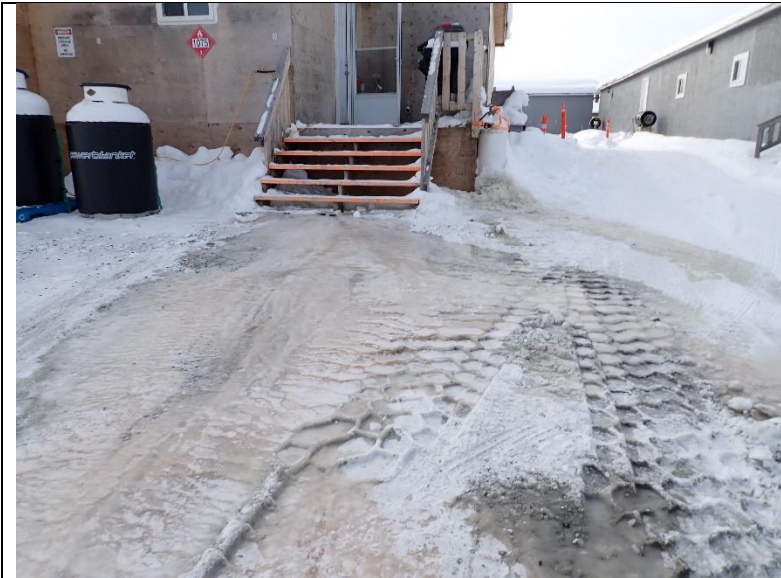
Photo #1: Overview of the back of the kitchen building, where a frozen and damaged pipe has resulted in grey water discharge and subsequent icing.
