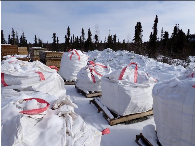
Photo #6: Waste material staged at the end of the airstrip in preparation for backhaul on the winter road and appropriate disposal. All materials were securely packaged, labelled, and weighted.
