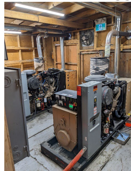
Figure 9: 75Kw and 100 Kw John Deere diesel generators.
