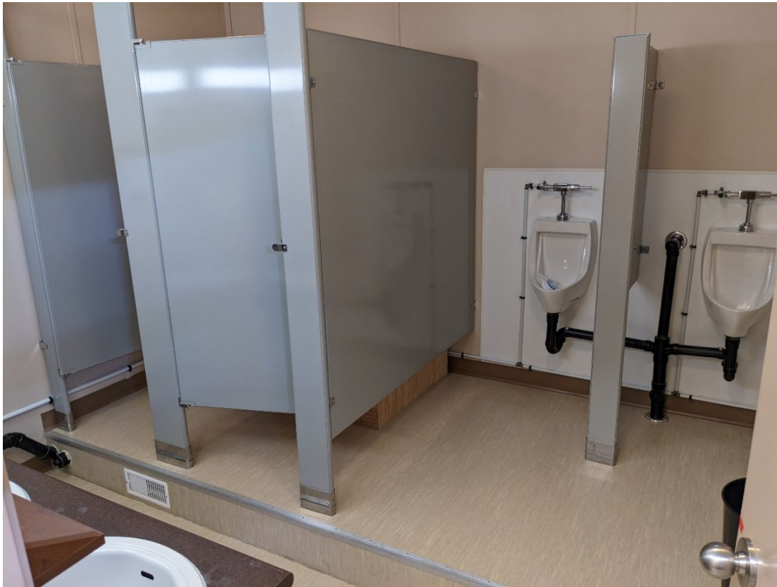
Figure 25: Dormitory communal washrooms with urinals, sinks, and toilet stalls (2023).
