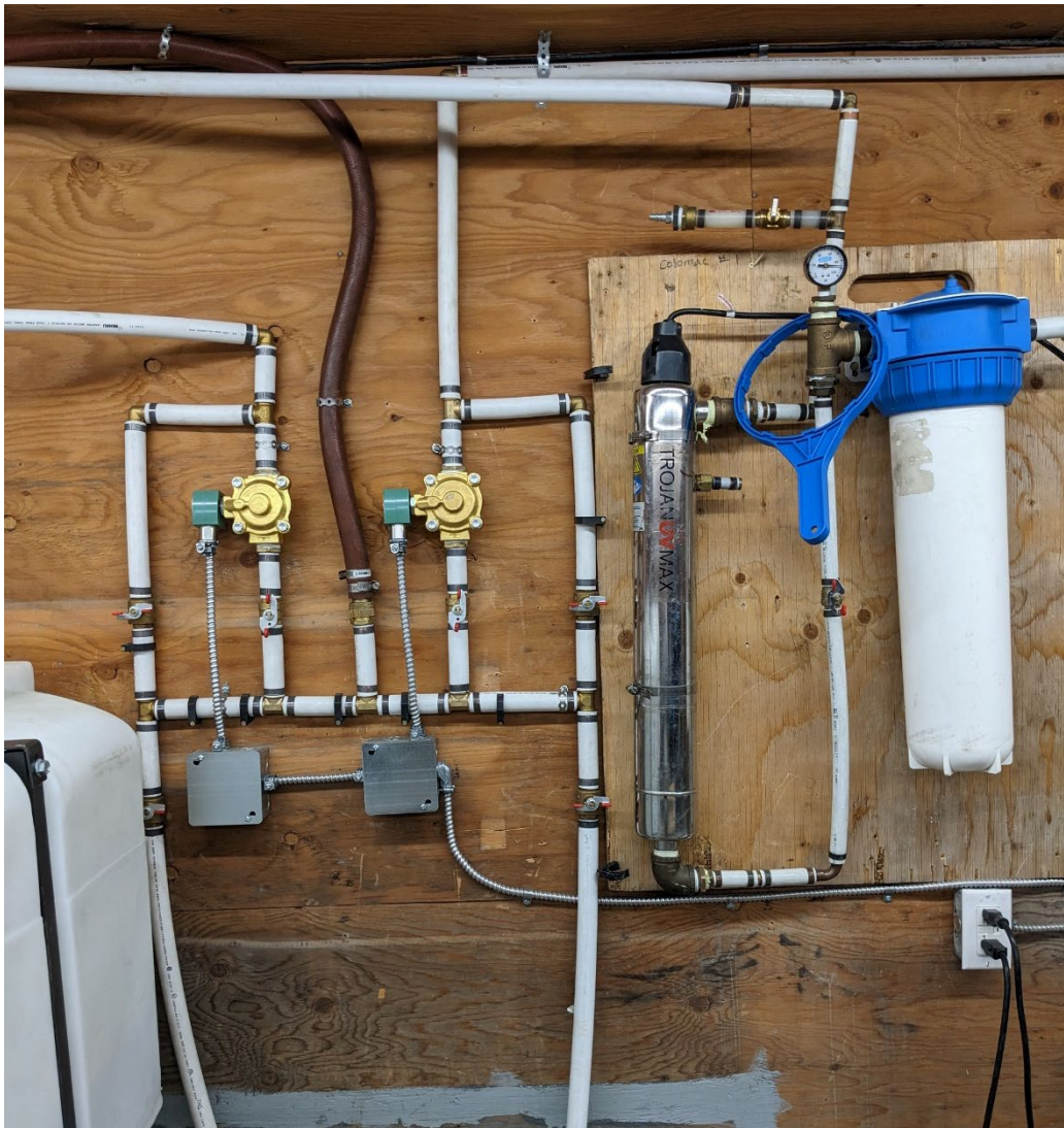
Figure 32: Water tanks fill control board (2023).
