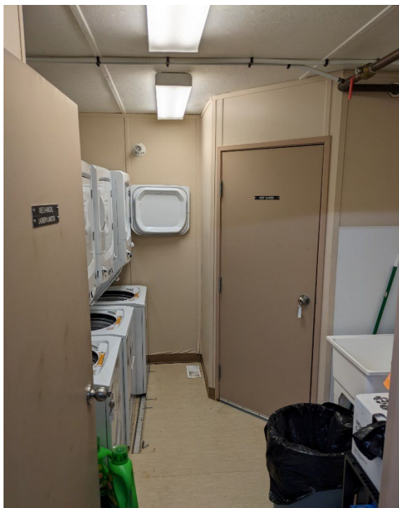
Figure 23: Dormitory trailer laundry room with washer-dryer combo machines on the left and door to hot water heater straight ahead (2023).
