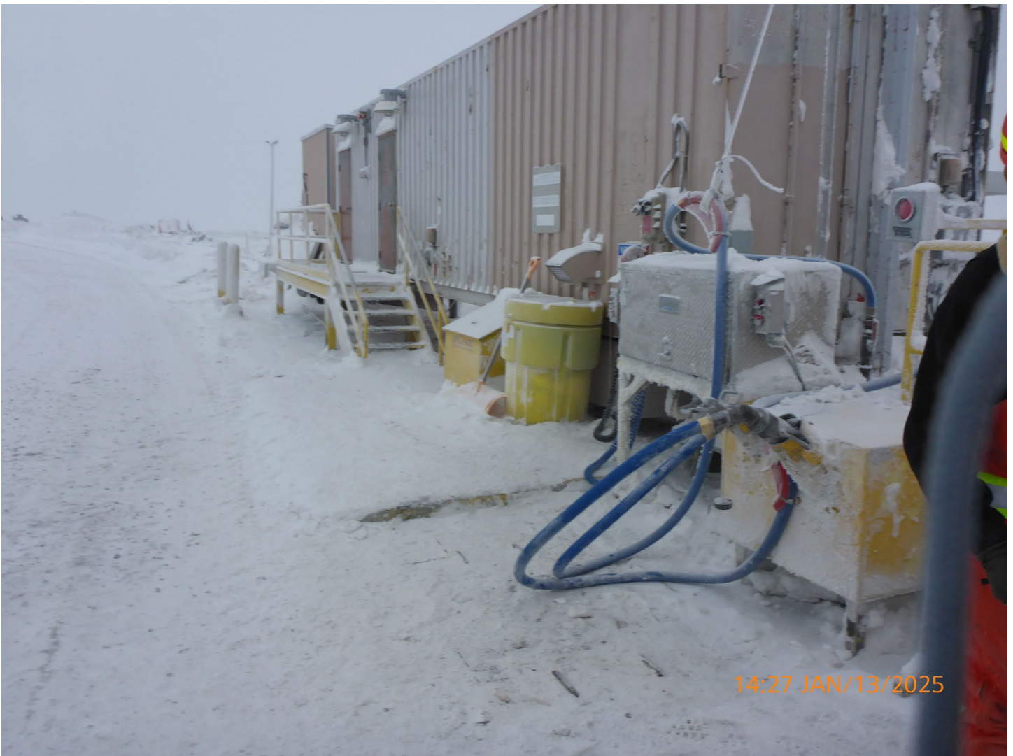
Photo 4 – Koala Refuelling – The Koala Refuelling Station was clean and well organized with no indication of any leaks or spills.
