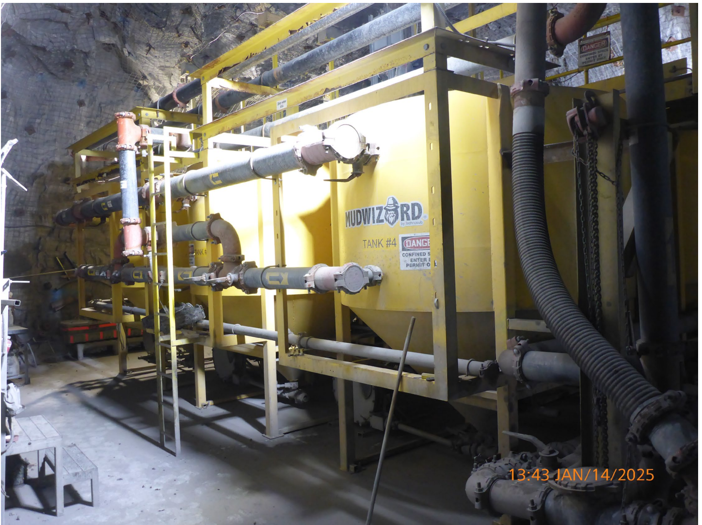
Photo 22 – Misery Underground – The Mud Wizard treats underground water to remove suspended solids. The water is then reused for mining equipment or sent to the surface for disposal in King Pond or Lynx Pit.
