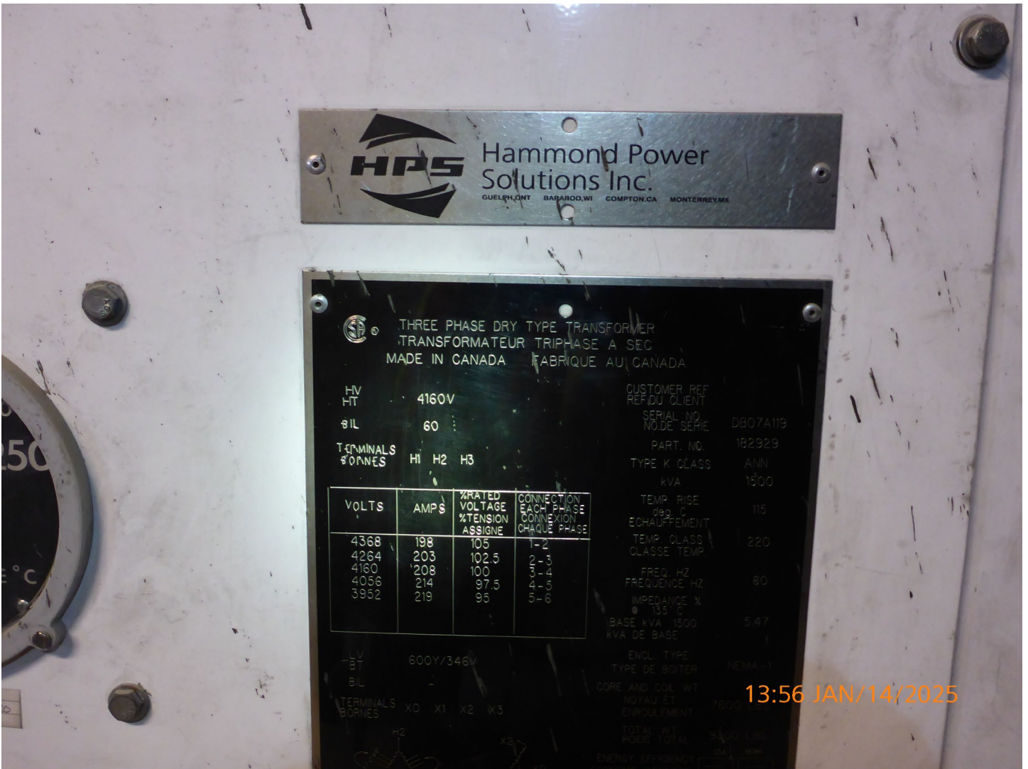
Photo 25 – Misery Underground – Transformers used underground are “Dry Type” and don’t use or contain any oils that can potentially contaminate water if flooded.
