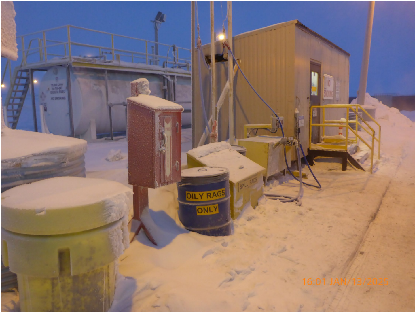
Photo 1 – Main Camp Refuelling – The Main Camp refuelling area was clean and well maintained with no indication of any hydrocarbon leaks or spills.
