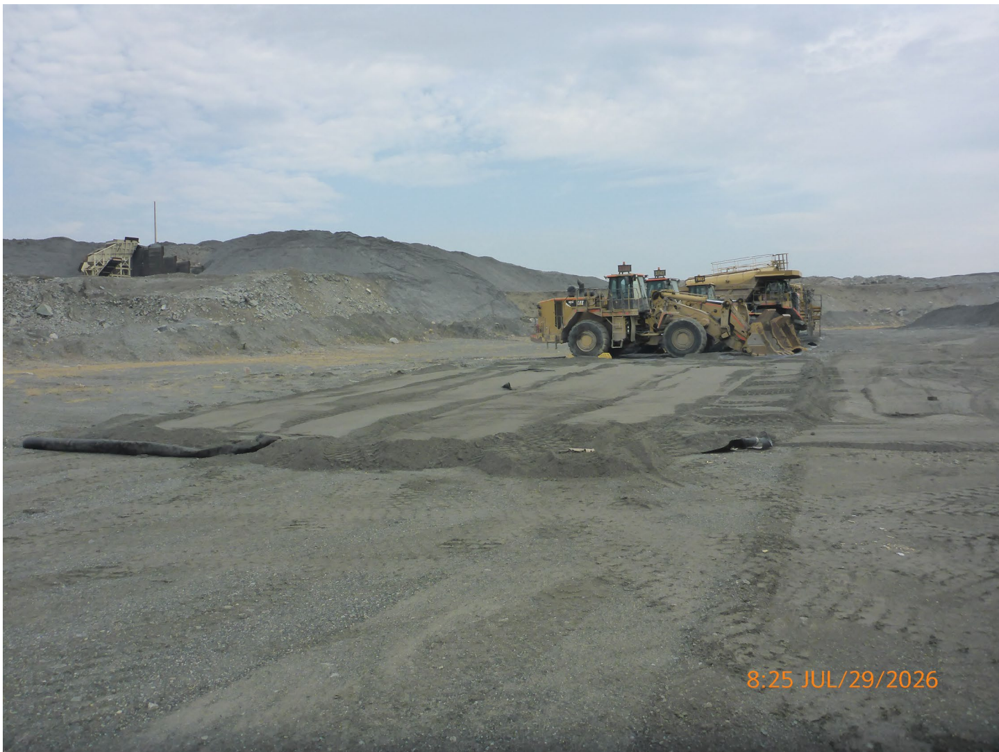
Photo 8 – Zone 12 – Lined parking areas have been created to contain any potential hydrocarbon leaks or spills.
