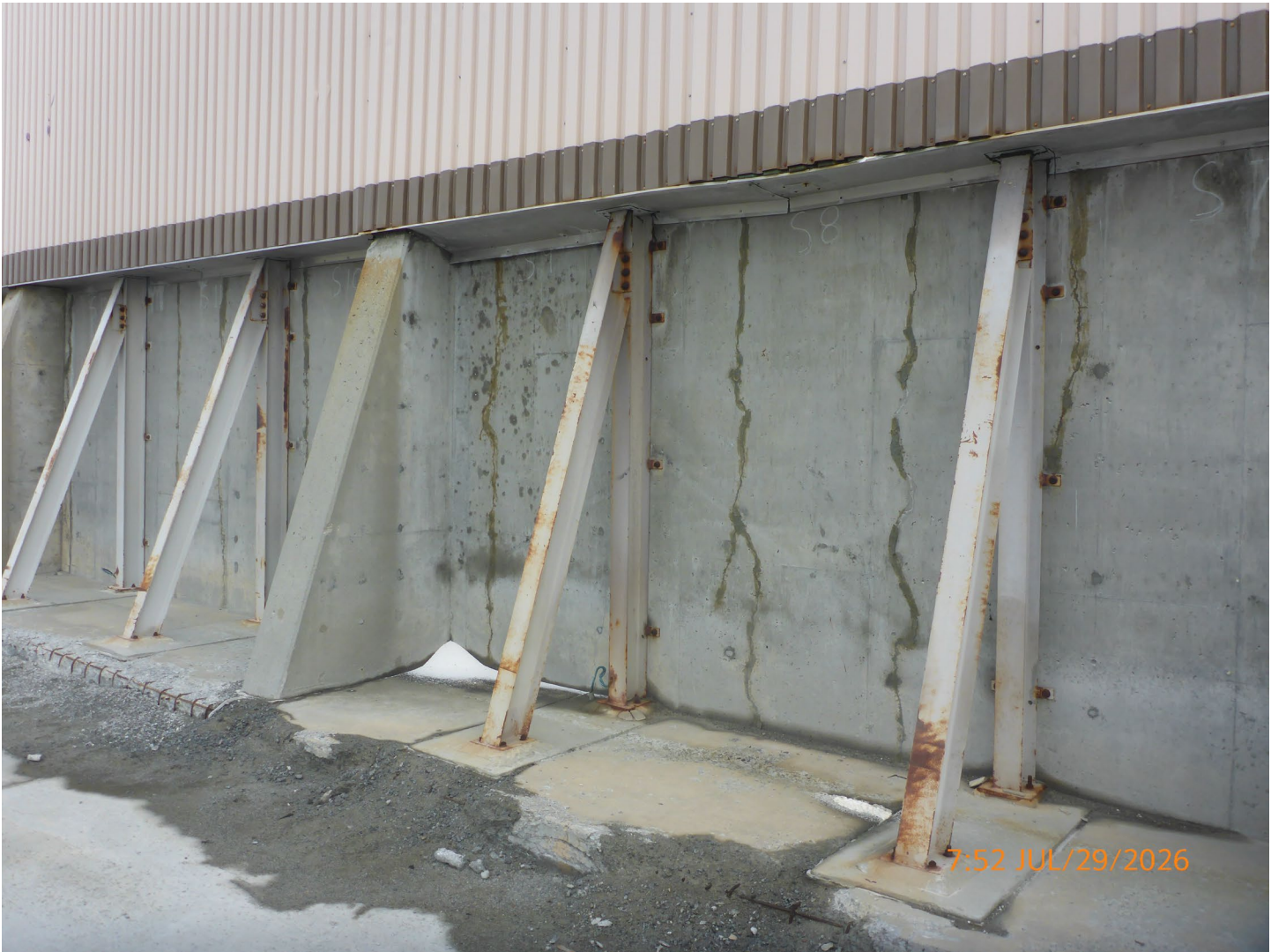
Photo 2 – Ammonium Nitrate Building – A small amount of AN is seeping though openings in the siding above the concrete containment at Section S8 on the southern wall of the building.
