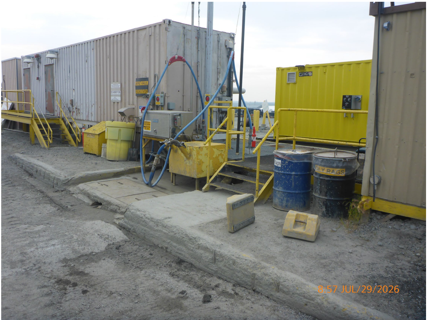
Photo 14 – Koala Heavy Equipment Refuelling – The Koala Heavy Equipment Refuelling station was clean and well maintained. Spill response equipment was fully stocked and easily accessible.
