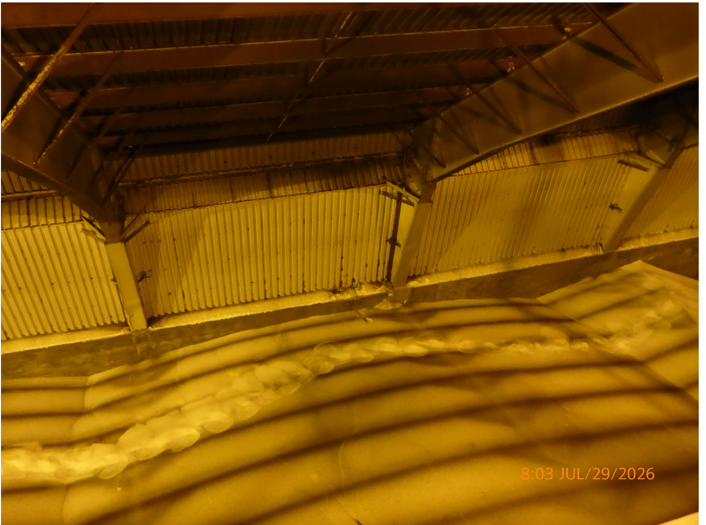
Photo 5– Ammonium Nitrate Building – The Ammonium Nitrate storage levels are below the concrete containment, however, dust has accumulated along the top of the concrete containment and is in contact with the metal siding causing corrosion.
