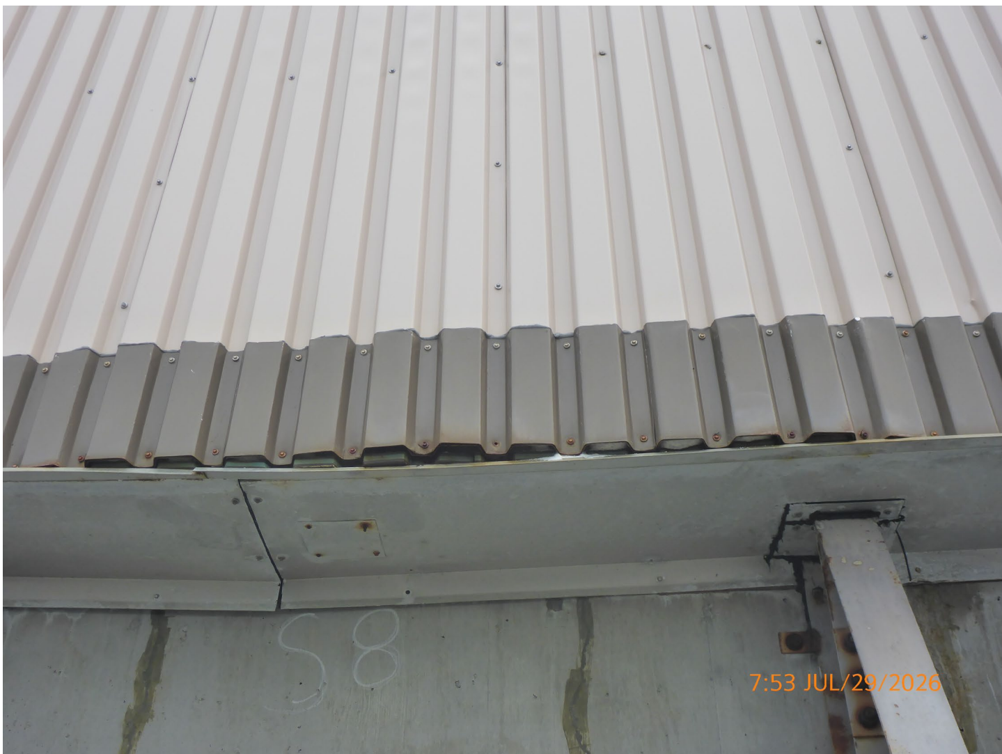
Photo 3 – Ammonium Nitrate Building – AN dust along the concrete containment is causing corrosion of the metal siding allowing AN to seep through.
